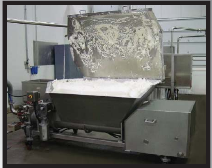
A 2000 Pound Batch of Sandwich Cream Filling in a RAM™ Pump Feeder Hopper (the pump feeder is connected to the production system via stainless steel piping)
