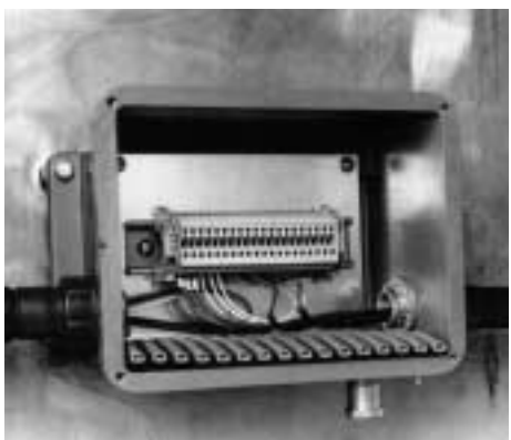
Electrical terminations in NEMA 4 enclosures with drip drains at low points and rubber mats to insure wires are kept away from standing water
